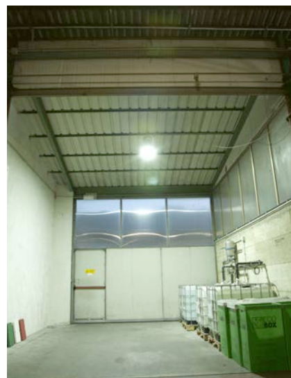
Warehouse illuminated with LED lamps. The illumination, at the same luminous flux, is more pleasant and shadows less accentuated.
